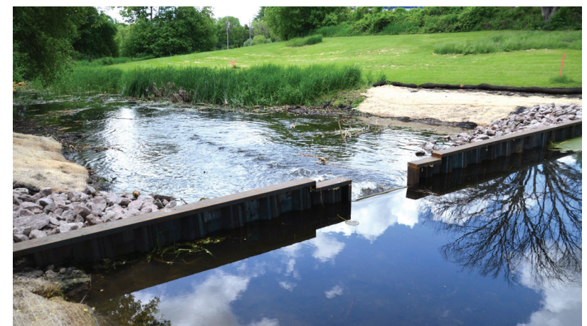
Last spring the ML-LPOA contributed $49,500 to build this weir across Mill Creek to maintain water quality and lake levels.
